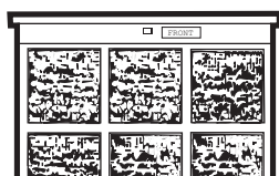
Dirty filter—Needs cleaning
